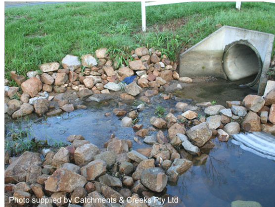
Photo 2 – Rock pad outlet structure
