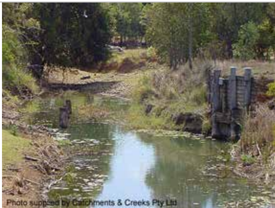
Incomplete removal of old bridge
