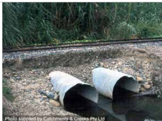
Flood damage to rail culverts
