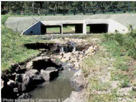
Head-cut erosion moving up to a culvert
