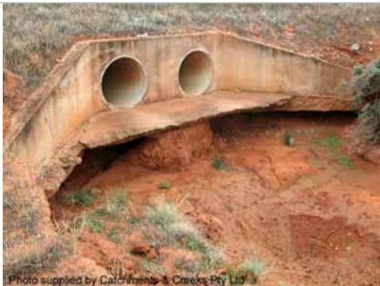
Outlet scour downstream of culvert
