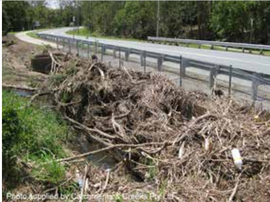
Debris blockage of culvert
