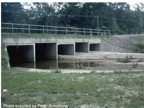
Culvert subject to heavy sedimentation
