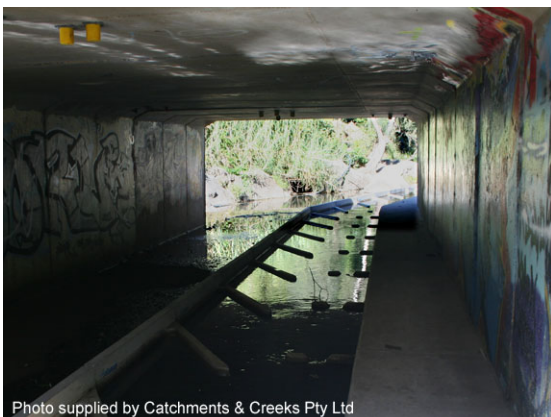
Offset floor baffles
