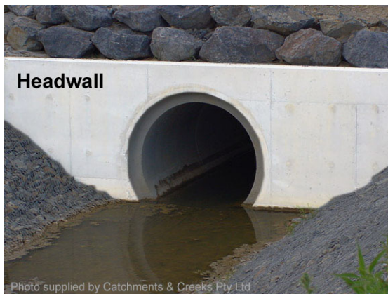
Culvert headwall without wing walls
