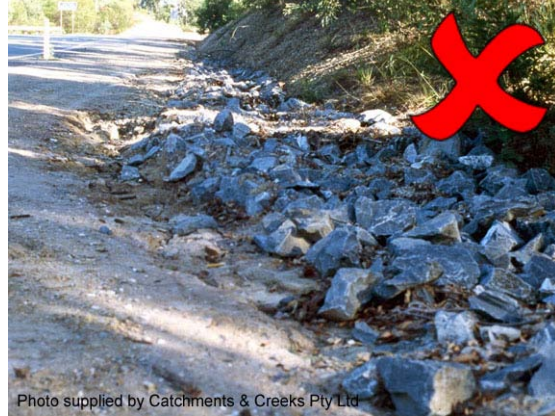
Photo 4 – In this example, placement of the rock has resulted in the rock-lined table drain being higher than the road shoulder
