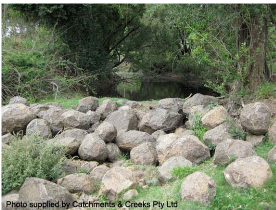
Photo 7 – Rounded rock can be significantly less stable than angular, fractured rock, especially when placed on steep slopes (Qld)
