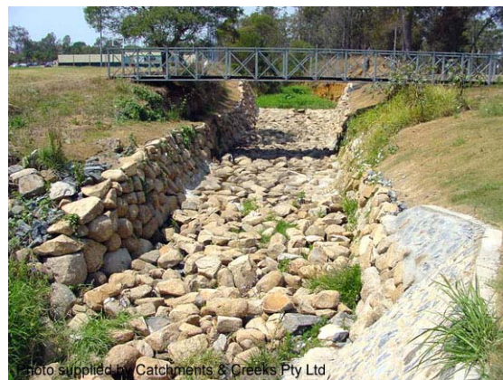
Photo 8 – Grouting boulders in place allows the use of smaller rock sizes in high shear stress chutes (Qld)
