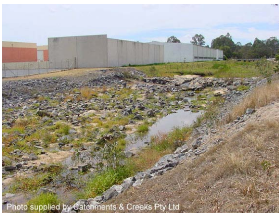
Photo 3 – Failed drop structure seven months after 1 in 30 yr storm
