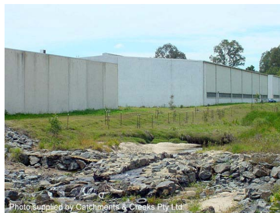
Photo 4 – Failed structure with concrete weir visible and undamaged
