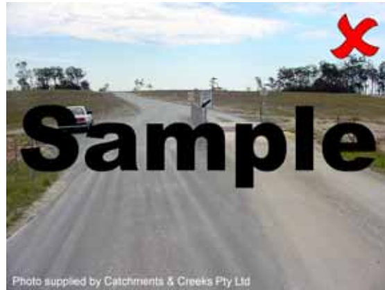
Photo 8 – Dividing site entry and exit lanes can result in vehicles bypassing the construction exit
