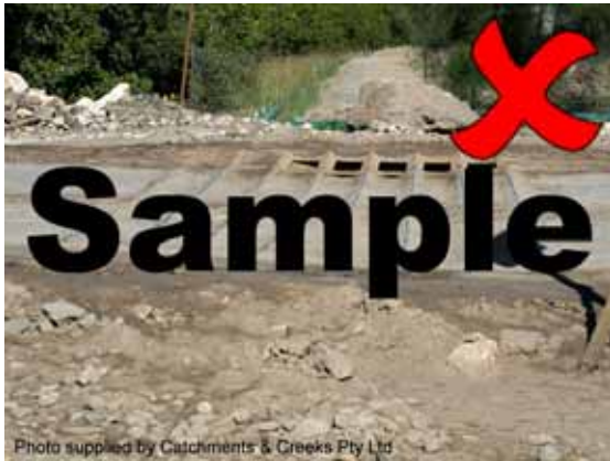
Photo 7 – Heavy sedimentation should not be allowed to occur at construction exits prior to their maintenance
