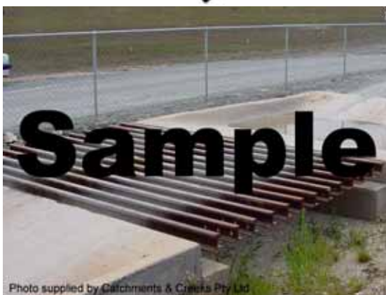
Photo 5 – Vibration grids are usually located prior to a wash bay
