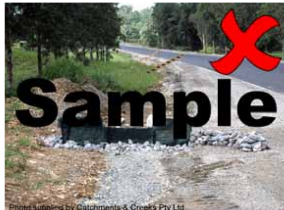
Photo 7 – This is not the correct structure for this application. The structure prevents the sediment from being collected.
