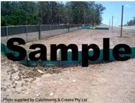
Photo 1 – U-shaped sediment trap within a drainage channel
