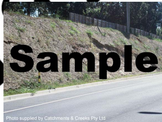
Photo 4 – Slippage of topsoil from steep cut batter
