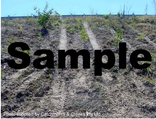
Photo 5 – Wheel track marks down a slope potentially causing concentrated runoff
