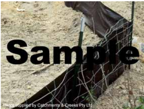
Photo 23 – Filtration with wire mesh
