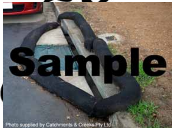
Photo 2 – side-entry kerb inlet (use of sediment trap)
