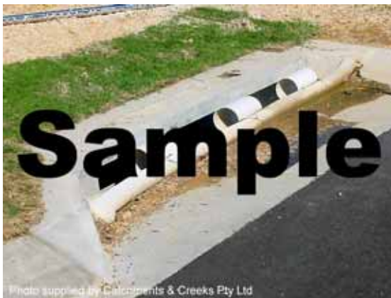
Photo 1 – side-entry kerb inlet (use of sediment trap)
