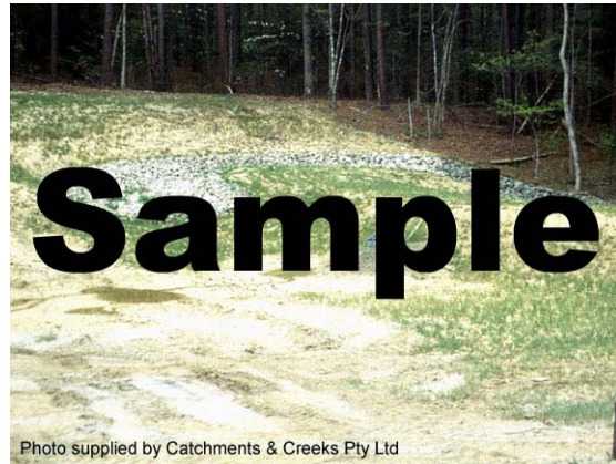
Photo 4 – Rock-lined spillway cut into virgin soil (note the spillway is curved up to the crest after which it remains straight)
