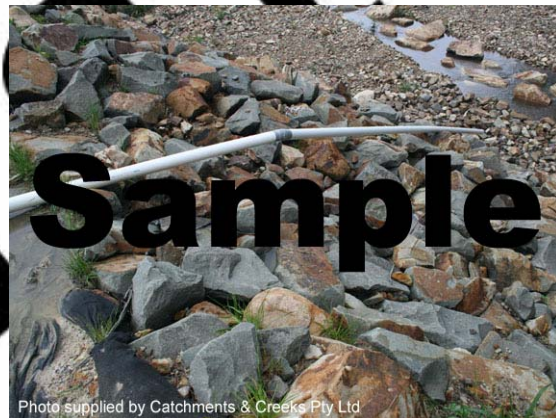
Photo 6 – Spillways lined with loose rock generally have a high risk of failure compared to concrete and rock mattress linings
