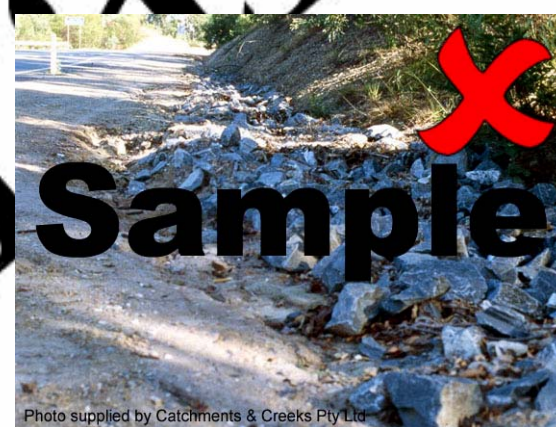
Photo 6 – In this example, placement of the rock has resulted in the rock-lined table drain being higher than the road shoulder
