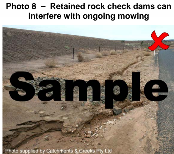
Photo 10 – Typical erosion problem when placed in dispersive soil
