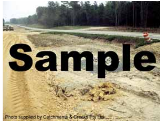
Photo 4 – Rock and aggregate drop inlet protection with optional sediment collection trench. Sediment collection trenches require attention.
