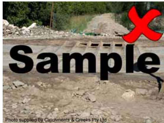
Photo 10 – Heavy sedimentation should not be allowed to occur at construction exits prior to their maintenance
