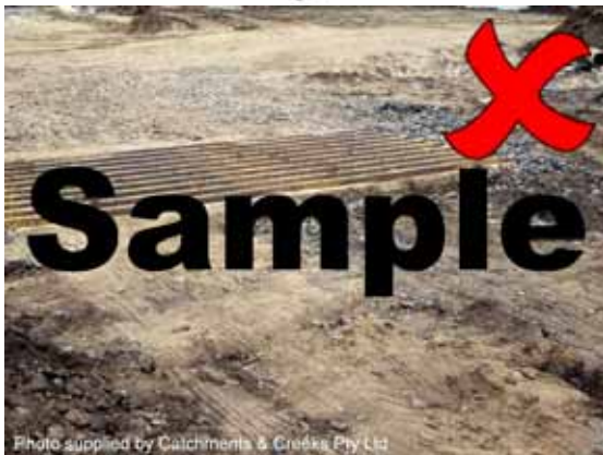
Photo 9 – Heavy sedimentation of rock pad adjacent a vibration grid
