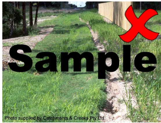
Photo 4 – Undesirable rilling along edge of turf caused by lateral inflows
