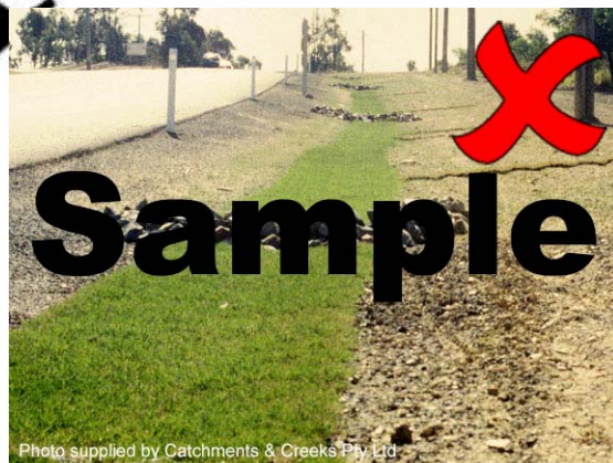
Photo 8 – Check dams and sediment traps placed on turfed drains can cause flow bypassing and erosion (rilling) along the edge of the turf
