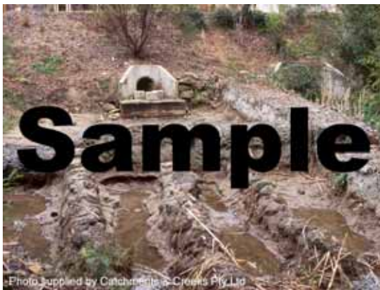
Photo 1 – Permanent excavated sediment trap at a stormwater outlet
