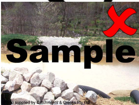
Photo 13 – Spillways must have a well-defined profile to fully contain the flow
