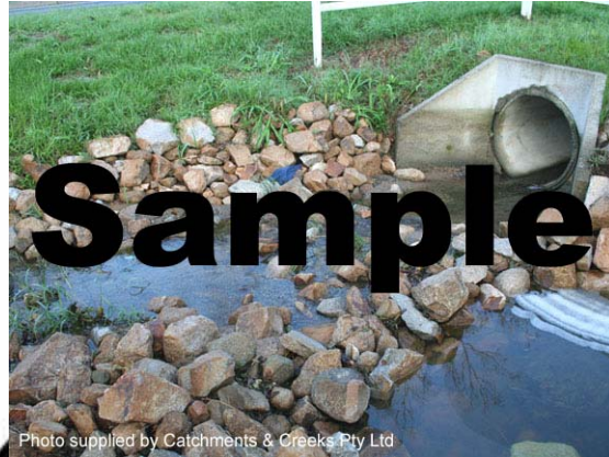
Photo 4 – Rock pad outlet structure
