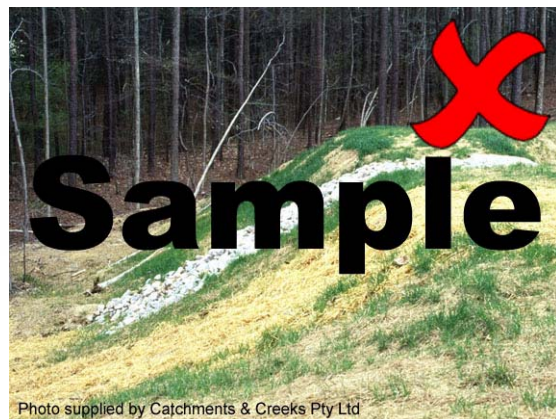
Photo 14 – A suitable energy dissipater must be constructed at the base of the spillway
