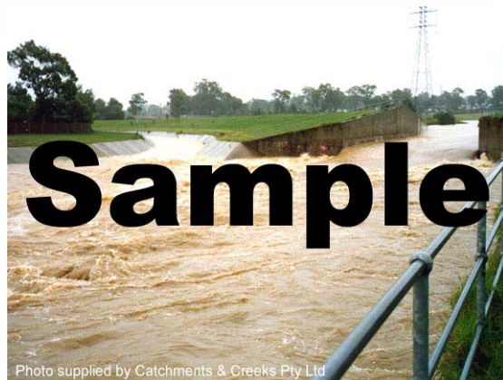
Photo 6 – Hydraulic jump dissipater downstream of detention basin outlet
