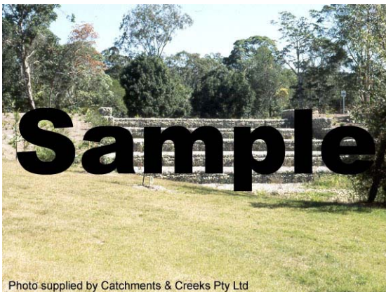
Photo 9 – Gabion lined stepped spillway on a stormwater detention basin
