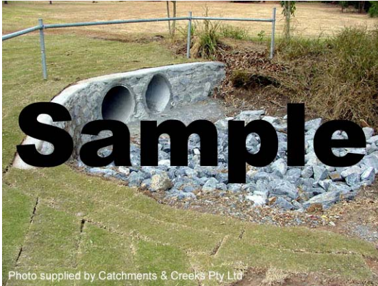
Photo 3 – Rock pad outlet structure
