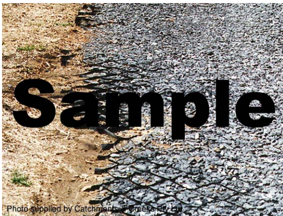
Photo 1 – Cellular confinement system used to restrict gravel movement on a permanent car park
