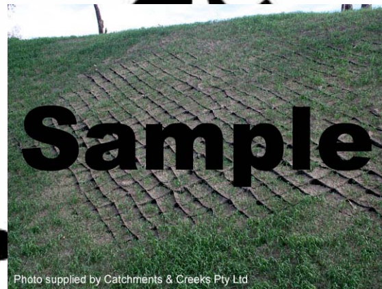
Photo 2 – Cellular confinement system used to retain soil and assist in the establishment of grass on a steep slope
