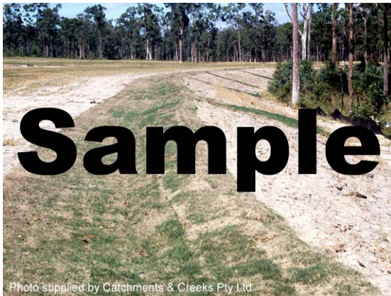
Photo 10 – Turf-lined flow diversion bank with grass-lined outlet chutes at regular intervals along the bankline
