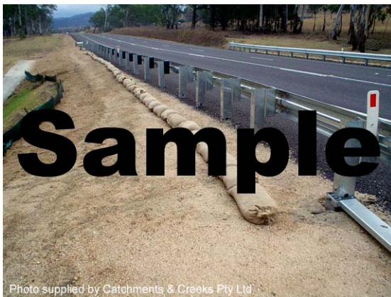
Photo 1 – Flow diversion berm used to minimise road runoff flowing down a steep, unstable section of embankment
