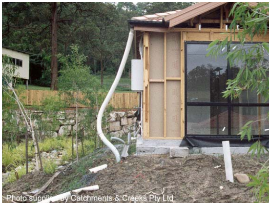
Photo 1 – Temporary downpipe (flexible pipe)
