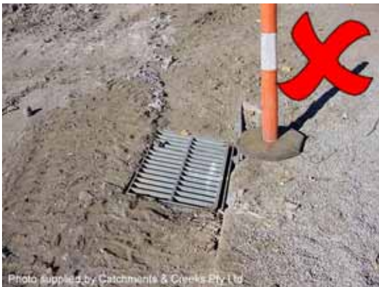
Photo 17 – No sediment control
