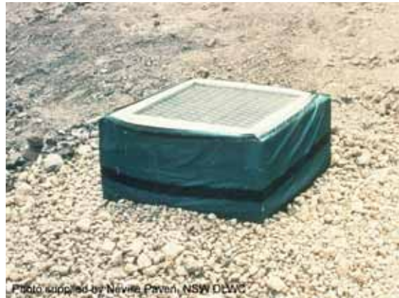
Photo 6 – Fabric drop inlet protection
