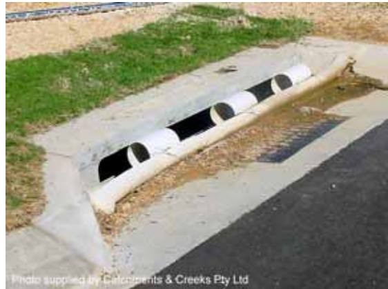
Photo 14 – Kerb inlet control system
