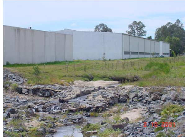
Photo 2 – Failed structure with concrete weir visible and undamaged
