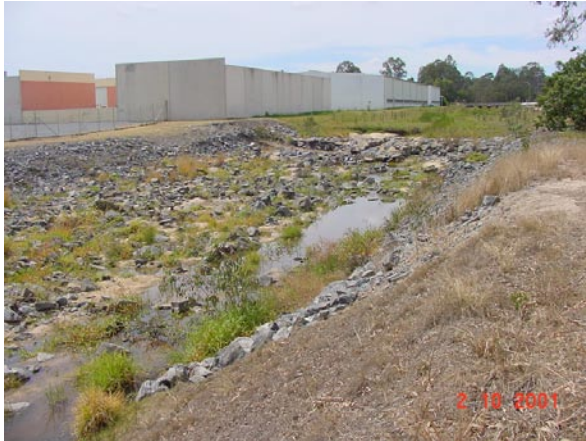
Photo 1 – Failed drop structure seven months after 1 in 30yr storm
